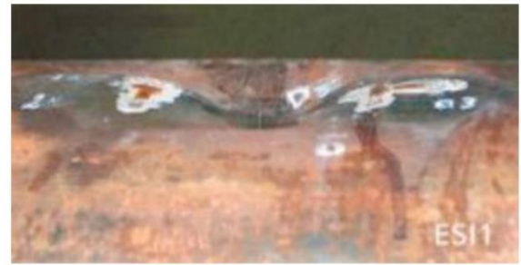
Figure 2. Dent in pipeline
