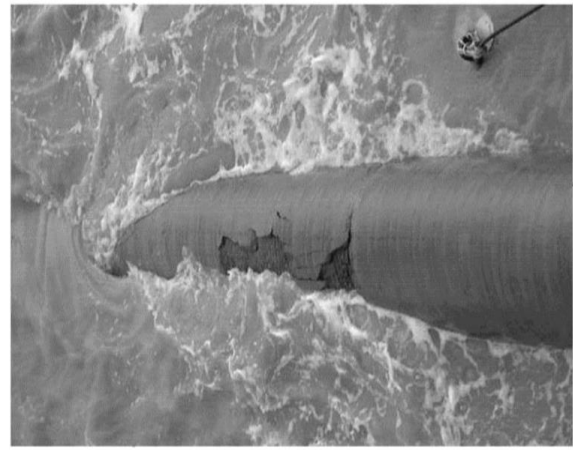
Figure 3. Crack in pipeline
