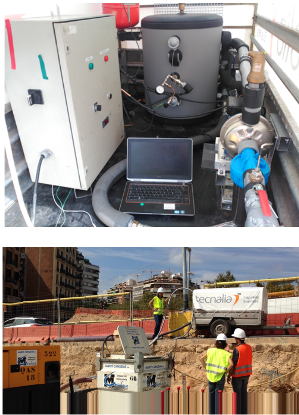
Figure 10. The Thermal Response Test equipment: The trailer installation (above), operation at Site A (below).
