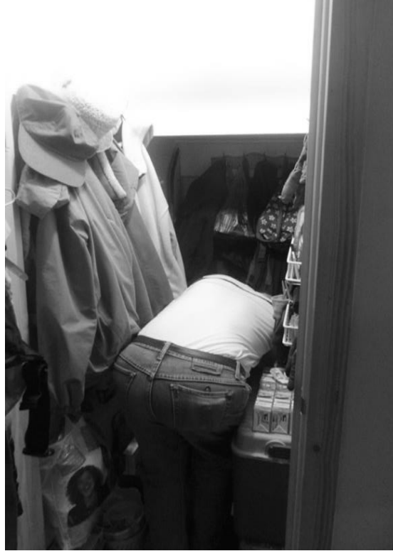
Figure 11. Poor location of the inverter (A)
