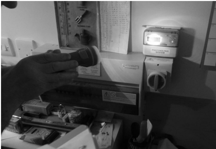
Figure 8. Poor illuminated display screen in the PV meter
