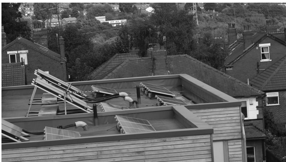
Figure 9. Inaccessible and hidden PV panels (A)
