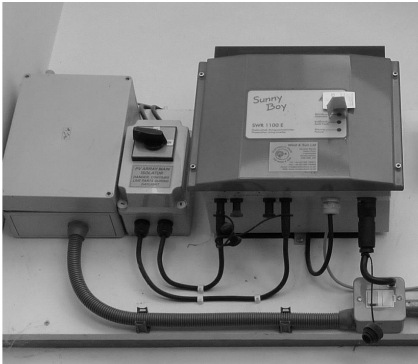
Figure 7. Poor provision of energy feedback in the installed inverter in case study C
