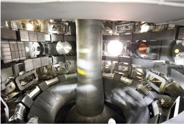
Figure 8: Photograph of the completed interior of MAST Upgrade prior to being pumped down.
