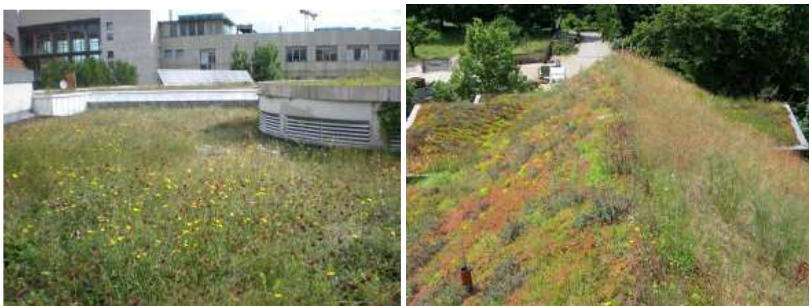
Figure 2. The roofs surveyed in Stuttgart included a) Rathausgarage complex and b) Killesberg.
