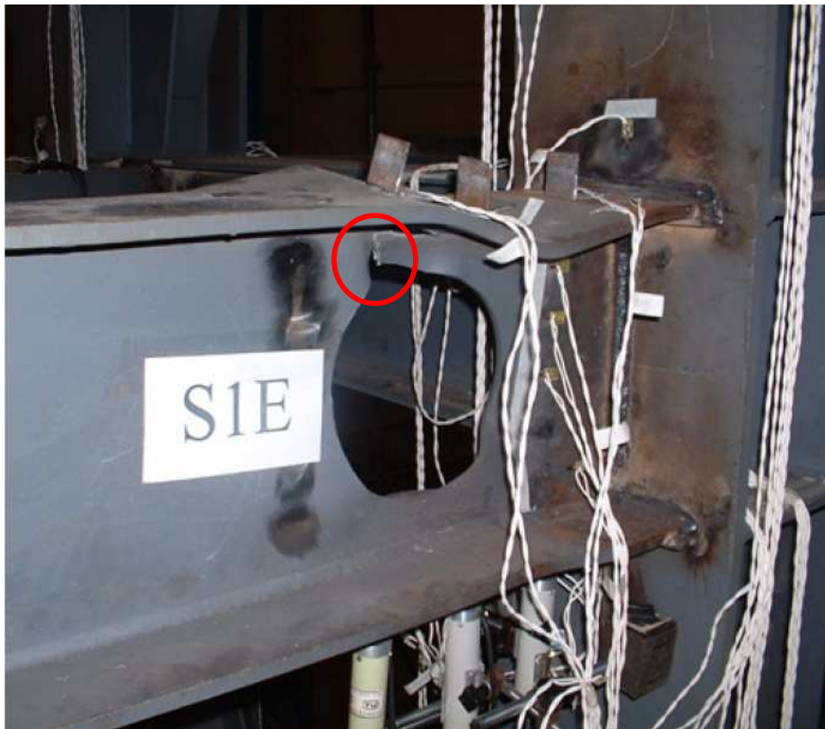
Figure 15. Failure mode of connection with web opening (Yang, et al., 2009)
