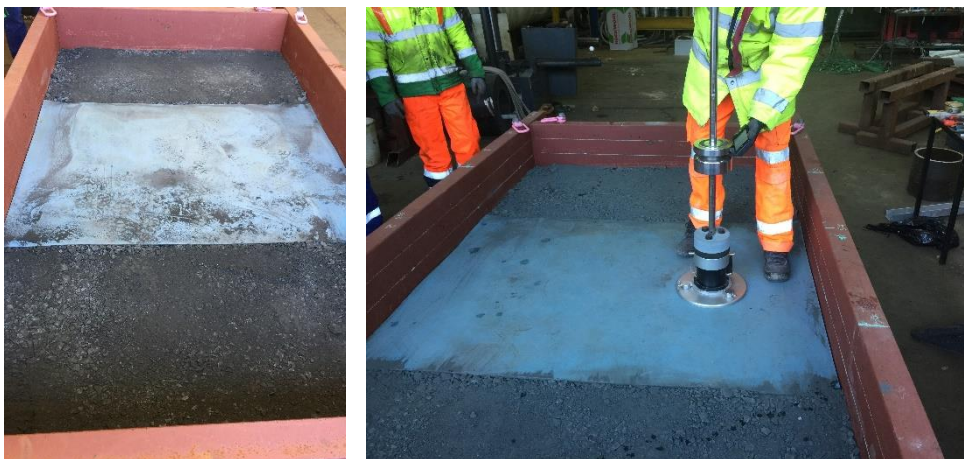
Figure 5. Compaction of sub-ballast (left) and Dynamic Plate Load testing using the LWD
