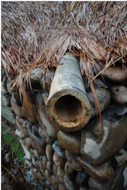
Figure 8. Bamboo drainage pipes directing rainwater from the thatched roof to the ground via stone foundation pads. Source: Sun Commune
