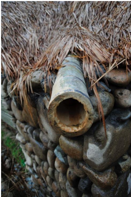
Figure 8. Bamboo drainage pipes directing rainwater from the thatched roof to the ground via stone foundation pads. Source: Sun Commune
