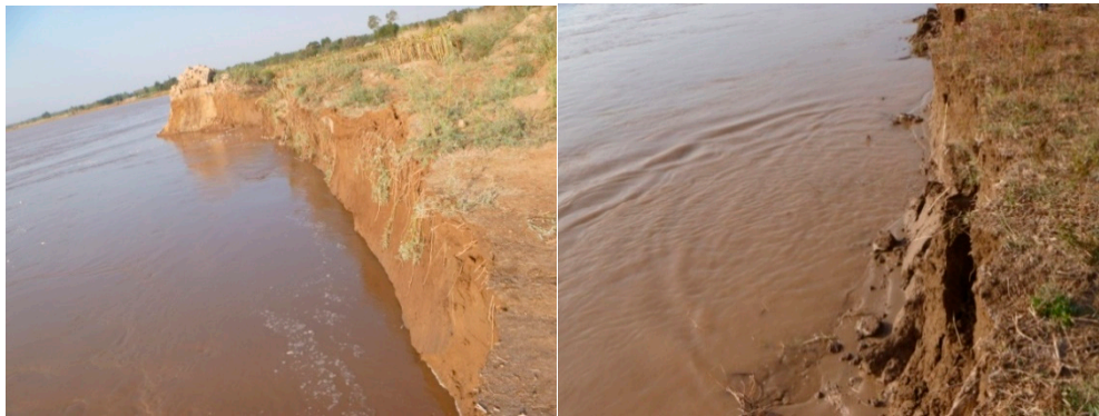
Figure 3. Example of the existing bank slope (left) and an example of riverbank collapse along Dengkou reach (right).
