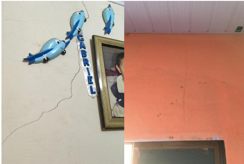
Figure 148 and Figure 149 - Cracks and leaking – House 03
