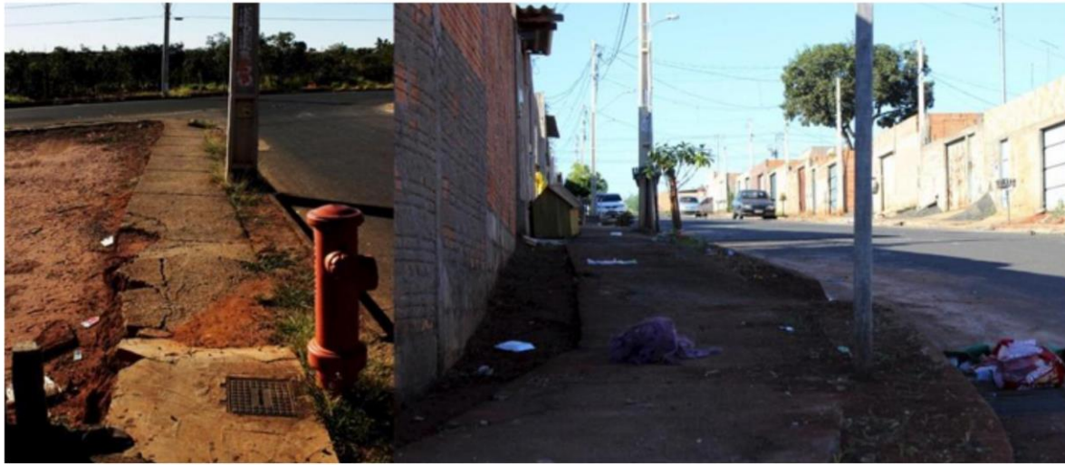
SIDEWALKS IN BAIRRO SHOPPING PARK - PROBLEMS WITH QUALITY AND MAINTENANCE
