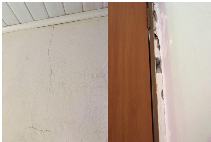
Figure 146 and Figure 147 - Cracks and leaking – House 02
