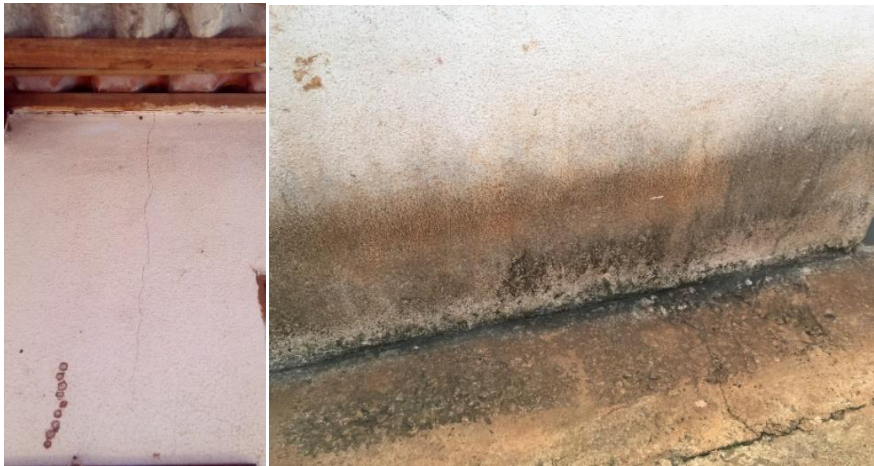
Figure 144 and Figure 145 - Cracks and leaking – House 01
