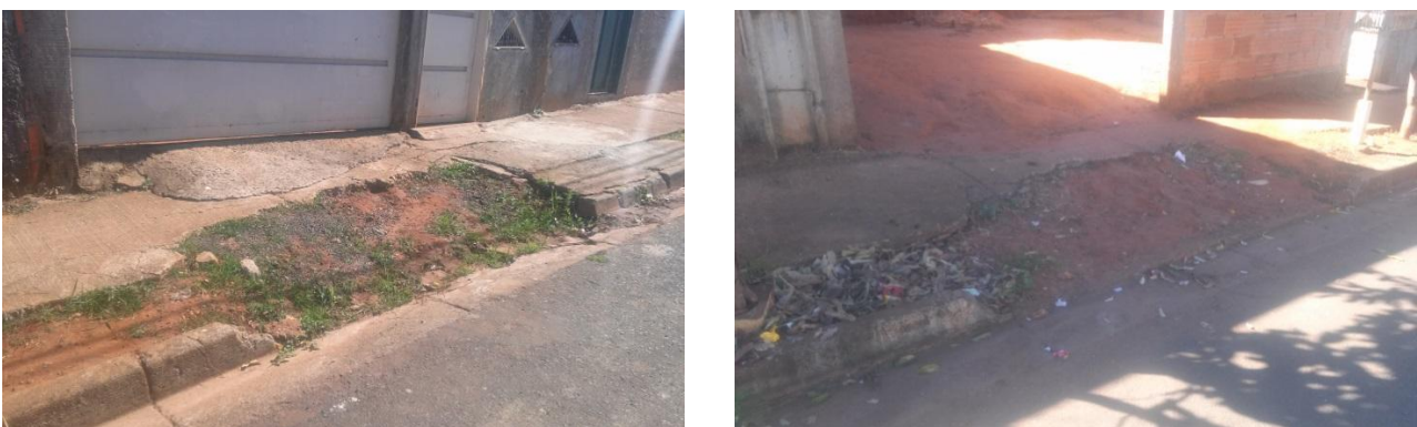
Figure 67 and Figure 68 - Broken sidewalks and car access ramp
