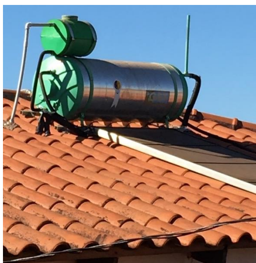
Figure 151 - Solar heating system and boiler on the roof – House 01
