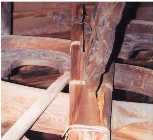
Figure 5 A column damaged due to an earthquake
