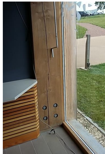
Figure 6 Vertical cracks occur in a column
