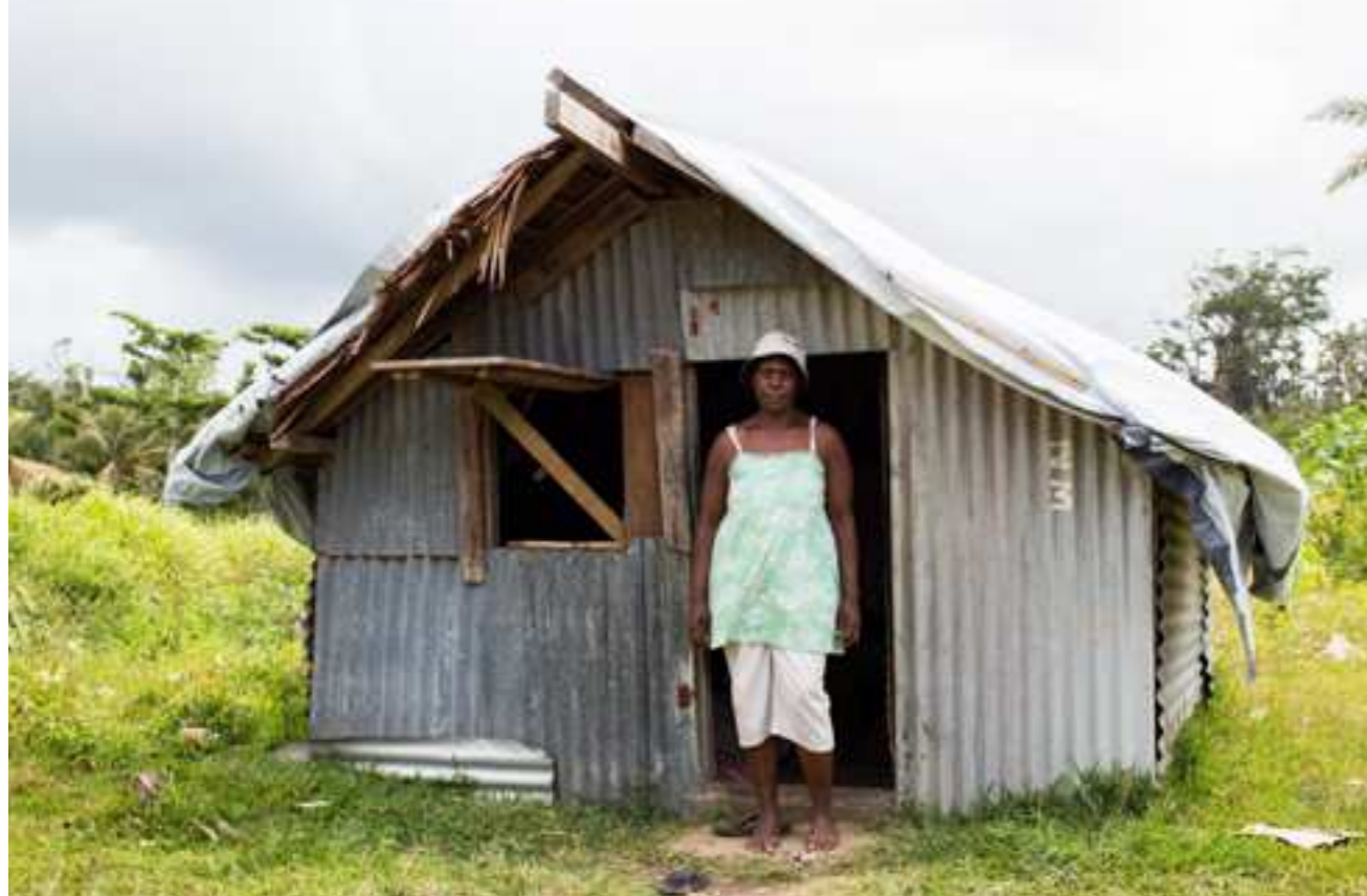
Six months after TCPam many homes remain under temporary repair. Photo: Arlene Bax/Oxfam
