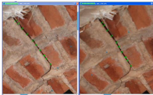
Fig 16. Non-targetted points of interest along a major crack used in photogrammetric measurement (Chen, 2014)
