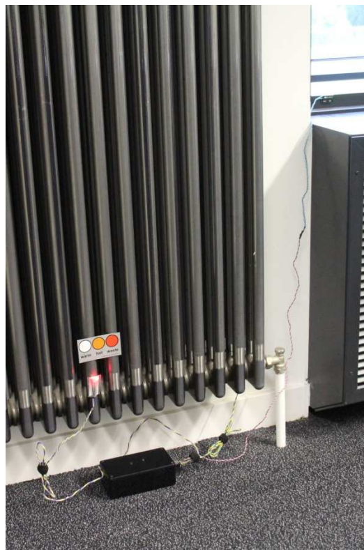
Figure 5.4 The radiator lights (feedback) attached to the radiator and window
