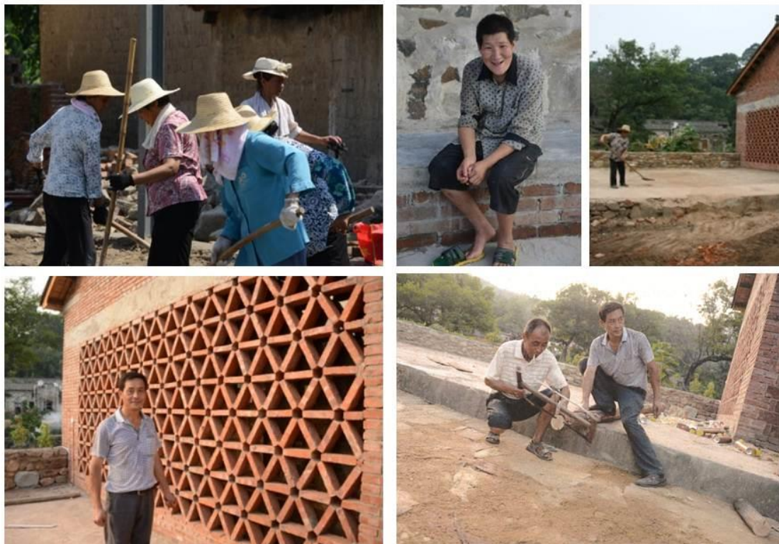
15 The construction team was made up of the remaining women, the disabled, the mason and the carpenter, all from the village. Summer 2014
