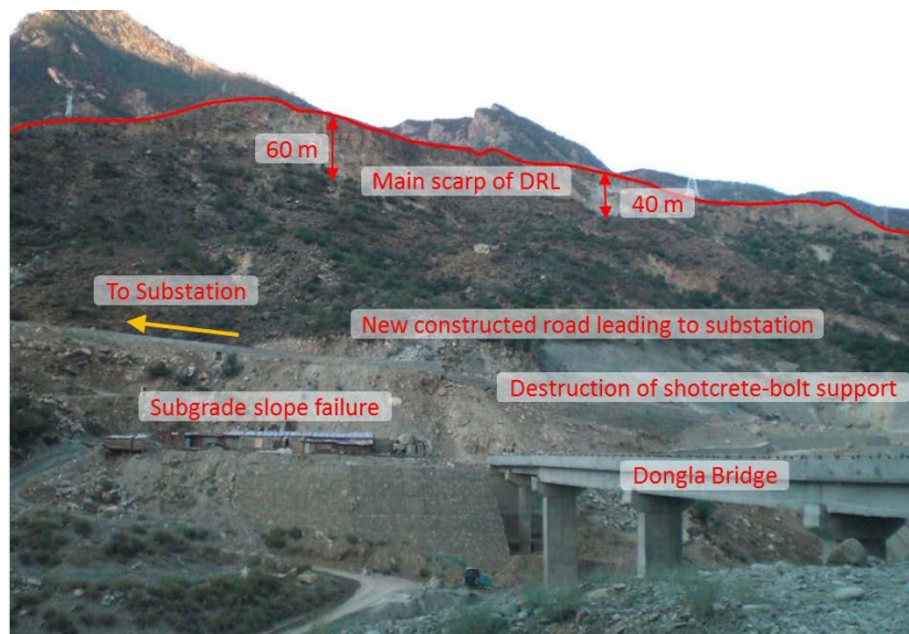
Fig. 6. Main scarp and local deformation features of the DRL. Viewing towards southwest.
