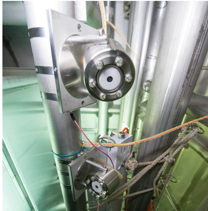
Figure 11. Two camera modules and mounts clamped to 3" SCH cryogenic pipes in the 35t cryostat.
