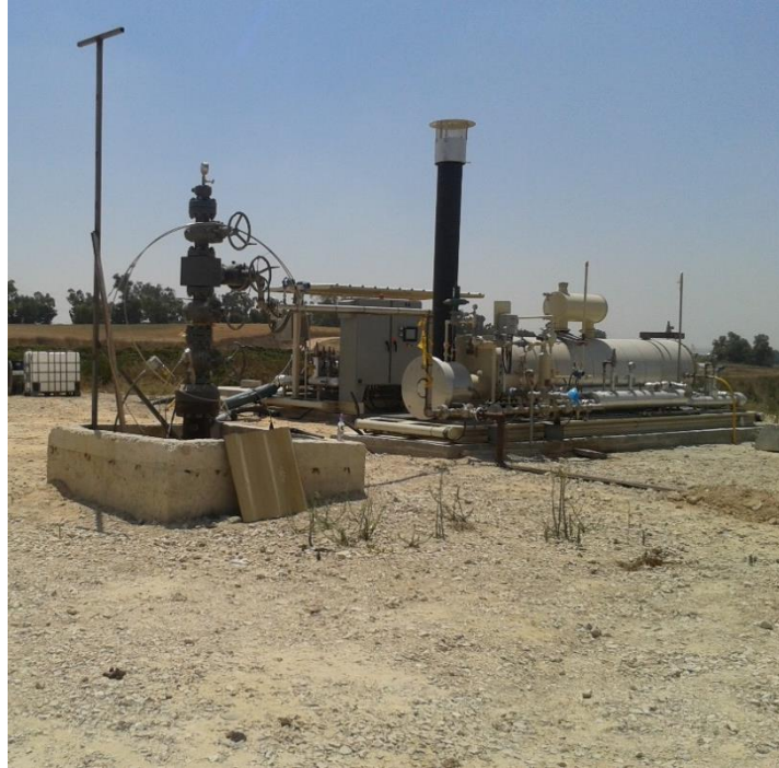
Figure 20. Connection to the injection well.
