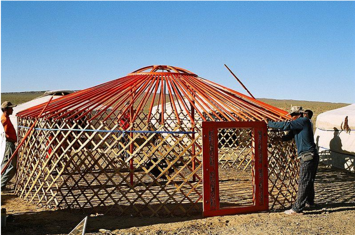
Figure 3: A ger under construction showing uni , toono , bagana and lattice frame panels. ( https://commons.wikimedia.org/wiki/File:Yurt-construction-2.JPG )
