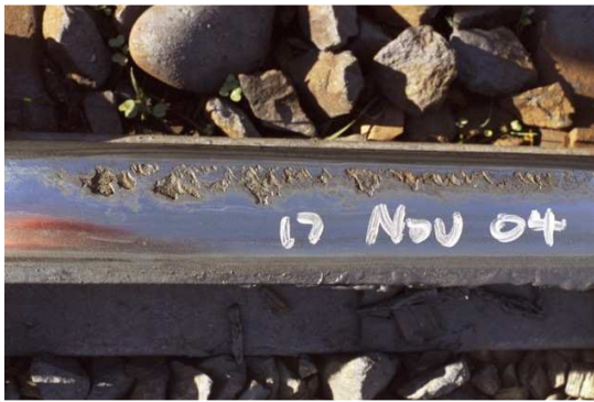
Figure 9: Example of spalling caused by an accidentally misplaced FM application unit in the spiral of a curve with pre-existing cracks on the rail surface. Optimized unit placement and corrective grinding prevented the problem from re-appearing.
