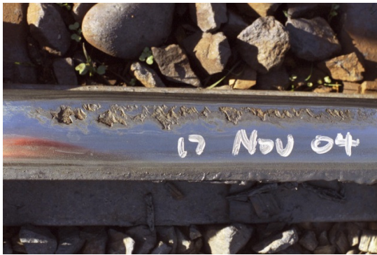
Figure 9: Example of spalling caused by an accidentally misplaced FM application unit in the spiral of a curve with pre-existing cracks on the rail surface. Optimized unit placement and corrective grinding prevented the problem from re-appearing.
