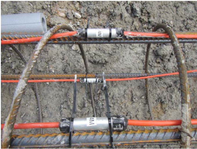
Figure 7. Detail of thermistor strings installed on the steel cage at 22 Station Road.
