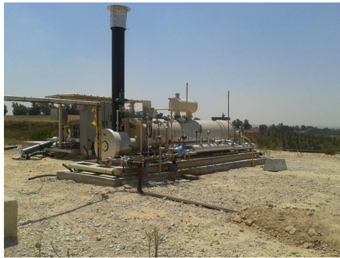
Figure 18. The heat exchanger.
