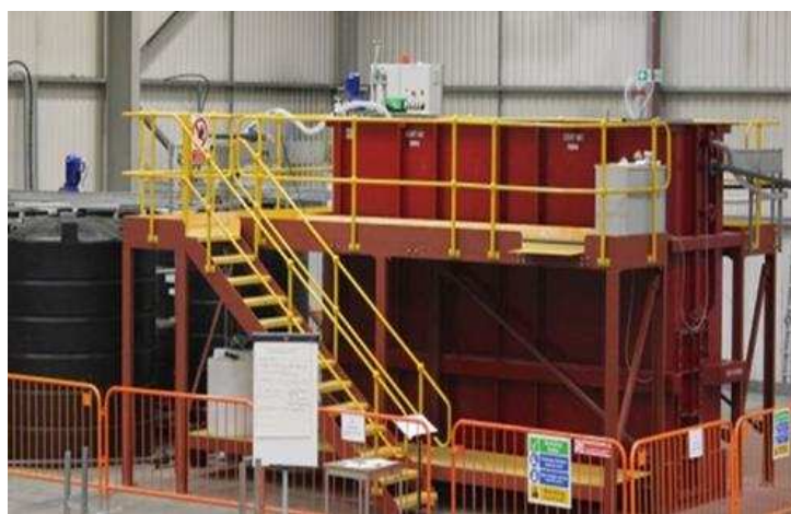
Figure 2: Image of large-scale settling clarifier at NSG Ltd, Chorley.
