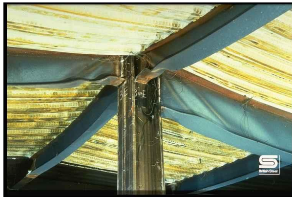
Fig. 1. Shear buckling phenomenon in Cardington Fire Test [2]
