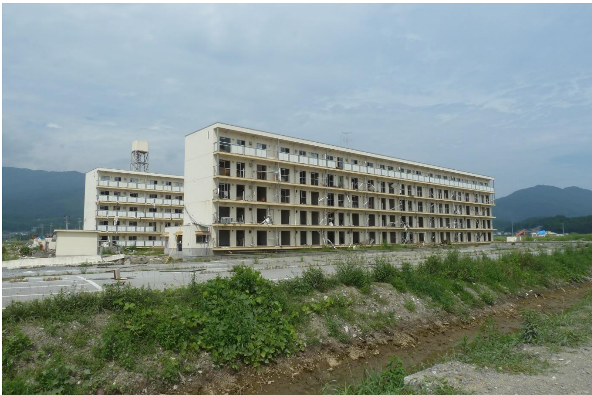
Figure 3. A destroyed warehouse for long term storage of frozen whale meat in the northern port area of Ishinomaki City, Miyagi Prefecture (August 2011).
