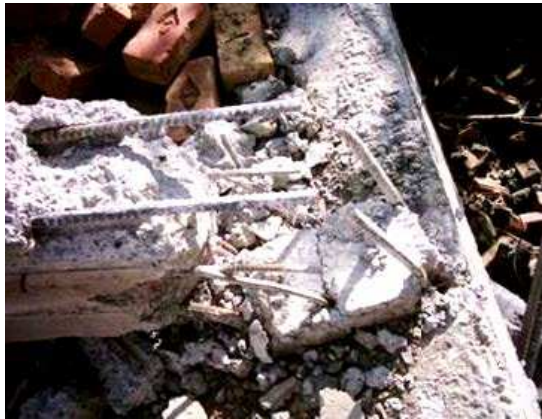
Fig. 1 Lap splice failure at the bottom of a RC column (2005 Kashmir earthquake; credit: S. Ahmad)
