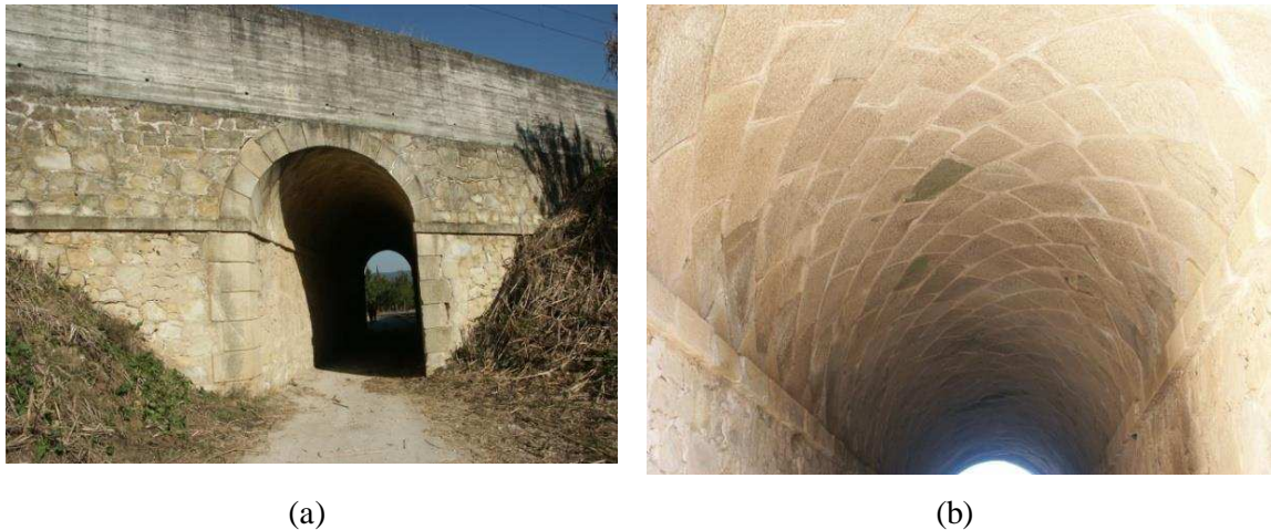
Fig. 1. Typical skew masonry arch constructed using the English method: (a) front view; (b) detail of the intrados
